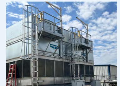
△ Cooling Tower operations at the Covington site have now been optimized, resulting in significant water and energy savings.
